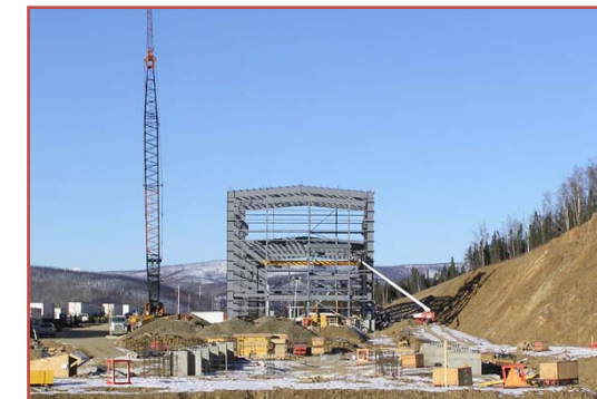
Sumitomo Metal Mining, Sumitomo Corporation, and Teck-Cominco have invested in the Pogo Gold Mine. Pictured: construction of the mill.
